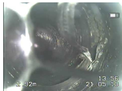
Figure 15 - Split chimney liner
