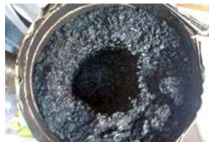
Figure 13 - Tared up chimney liner
