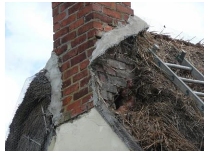
Figure 17 - Thatch by imperfect chimney brickwork
