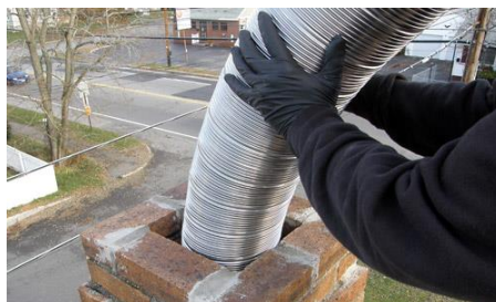
Figure 9 – Flexible lined chimney
